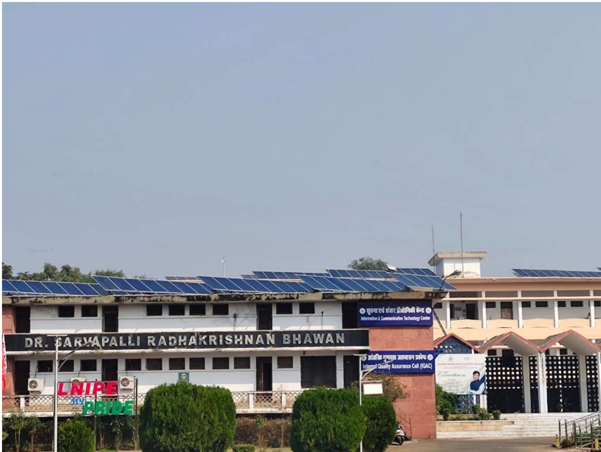
Figure 1 On-grid Solar power plant
